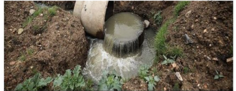
The sewage treatment plant section of the Vaal River.
